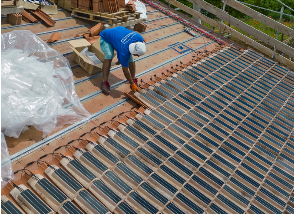
Province of Treviso (Italy). Laying a roof with roof tiles from the E-coppo company; the tiles have small photovoltaic panels inserted in them.
