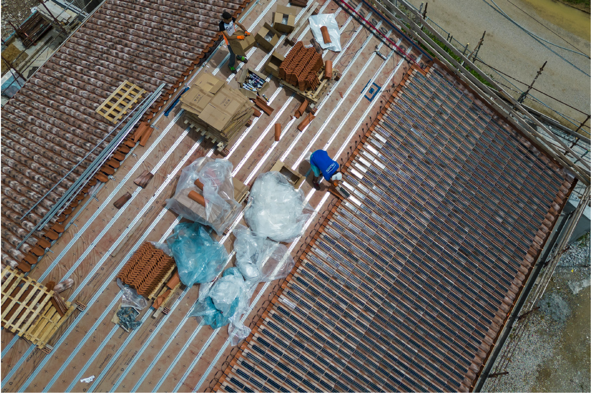
Province of Treviso (Italy). Laying a roof with E-coppo roof tiles that have small photovoltaic panels inserted in them.
