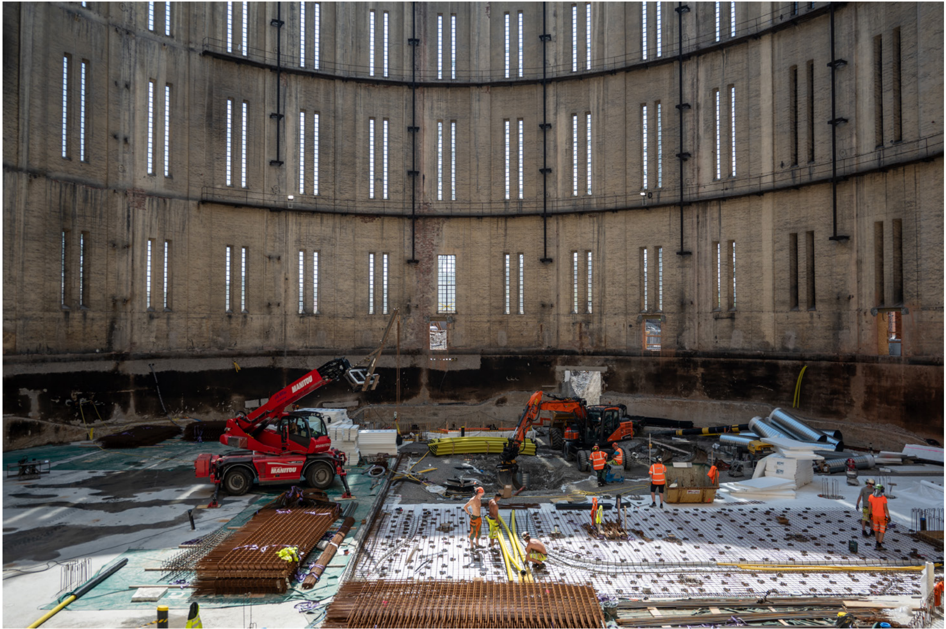
Stockholm (Sweden), renovation work at one of two "gasverkets," which used to store gas and will soon become a hotel and concert venue in the heart of the Stockholm Royal Seaport district.
