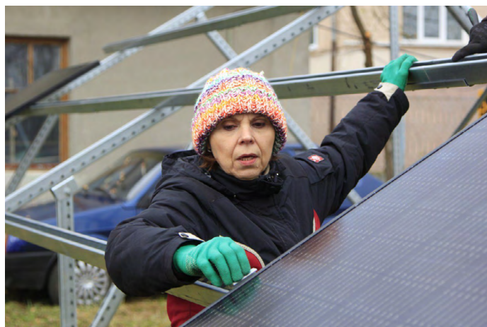
ECF partners Greenpeace Ukraine and RePower UA trained women to install photovoltaic solar panels while men fight in the ongoing war, which threatens critical infrastructure.
